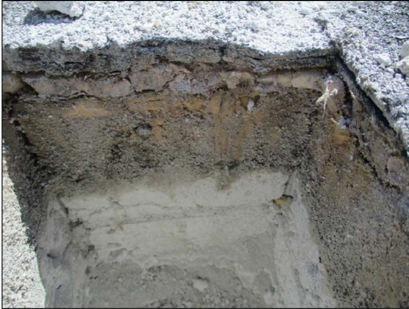
Photo 9: Core location R3, nuke reading 20 – moist conditions at Securock cover board and polyiso insulation boards.
