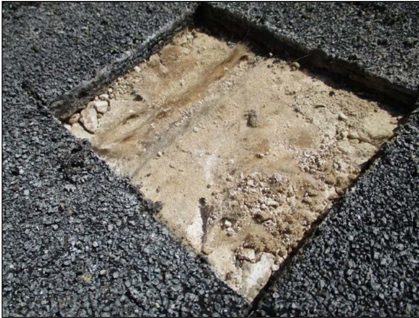
Photo 7: Core location R3, nuke reading 20 – cover board discoloration.
